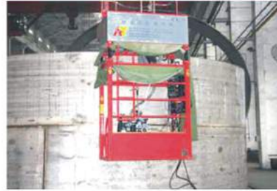
↑ 埋弧自动横焊机 (DN7200三聚氰胺反应器焊接中) Automatic Submerged Arc Welding Machine (DN7200 Melamine Reactor Under Welding)
